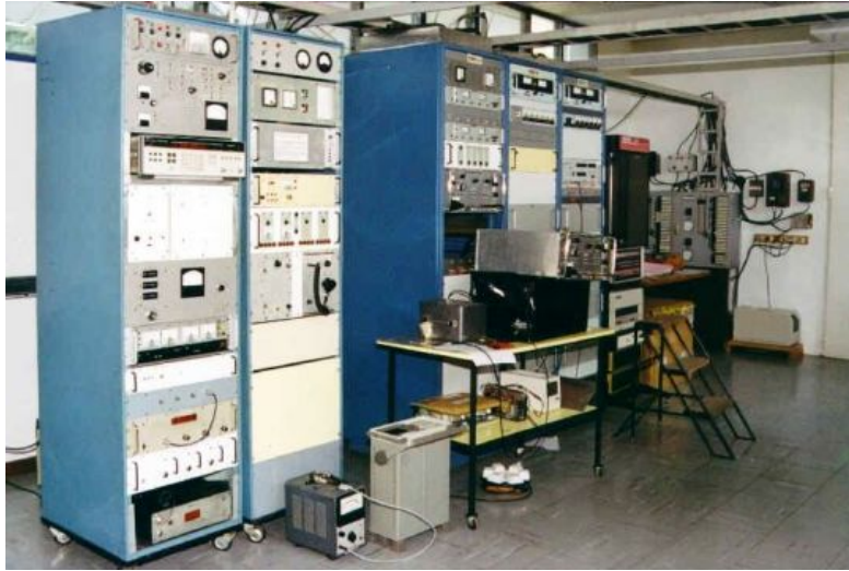
Panel de control - IAR
